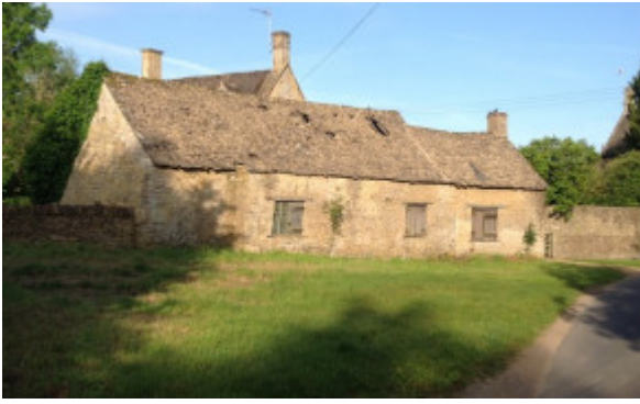
■ Derelict Barn at Broadwell
